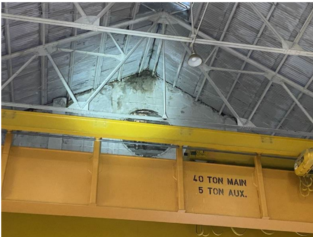
Figure 3-23. Staining under Roof at Main Entrance to the Powerhouse
